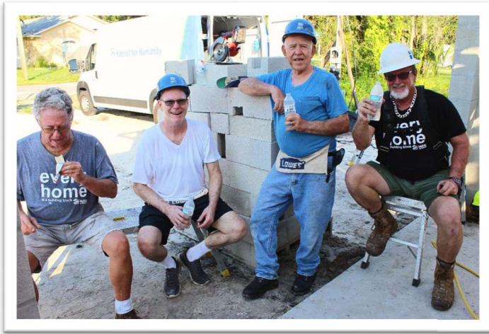
(L-R) Habitat for Humanity Wednesday Weekday Warriors Jeff, John, and PGK SK Jay Young take a much-needed break from doing roof truss fascia work on a house at 739 Alabama St. in Daytona Beach. Not pictured, Habitat Chairman Mark Leary, who was taking the photos.
