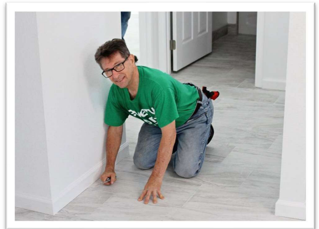
Trustee SK Russell Benett does some punch list item work on the baseboards at a house at 761 Alabama St. in Daytona Beach, which will be completed and dedicated on October 1.
